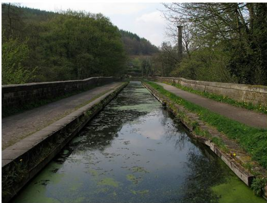
In this photograph you are looking across the Cromford aqueduct towards the Leawood Pump House. The distortion in the side walls of the structure is clearly apparent.
