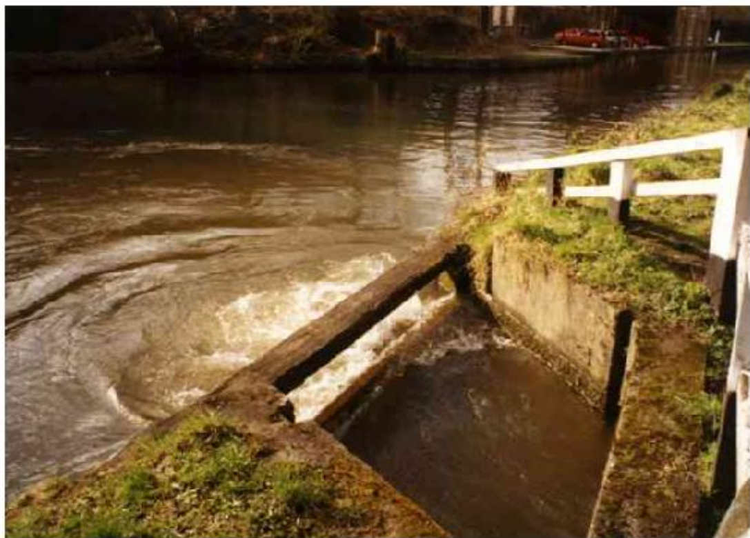
In this photograph, taken on one of the pump house running days, you can see the pumped water flowing out into the canal.
